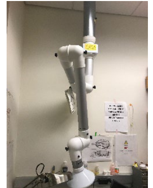
Image 11: Snorkel connected to the house exhaust ventilation
