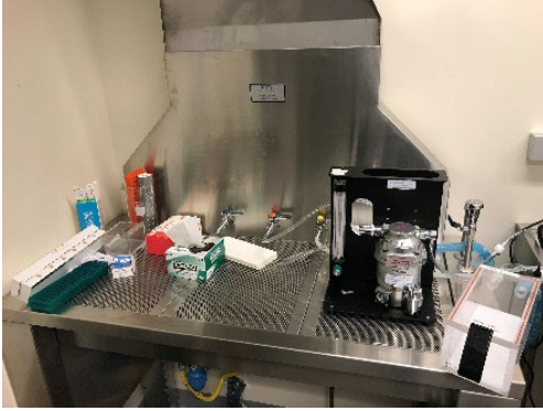
Image 9: Downdraft table connected to the house exhaust ventilation
